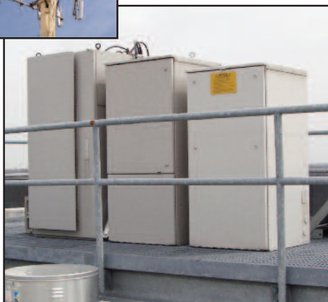
Typical Wireless Application
