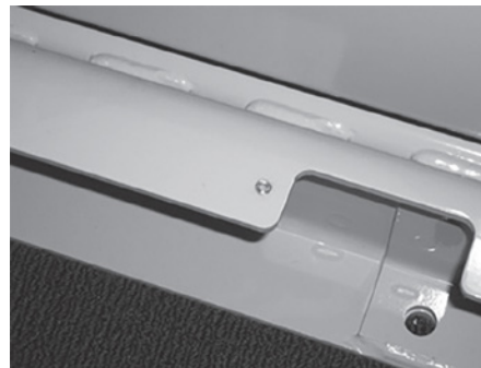
Figure 2: Adequate Paint Penetration
