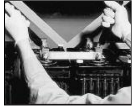
FIGURE 4.1.7 Measuring connection resistance with DLRO
